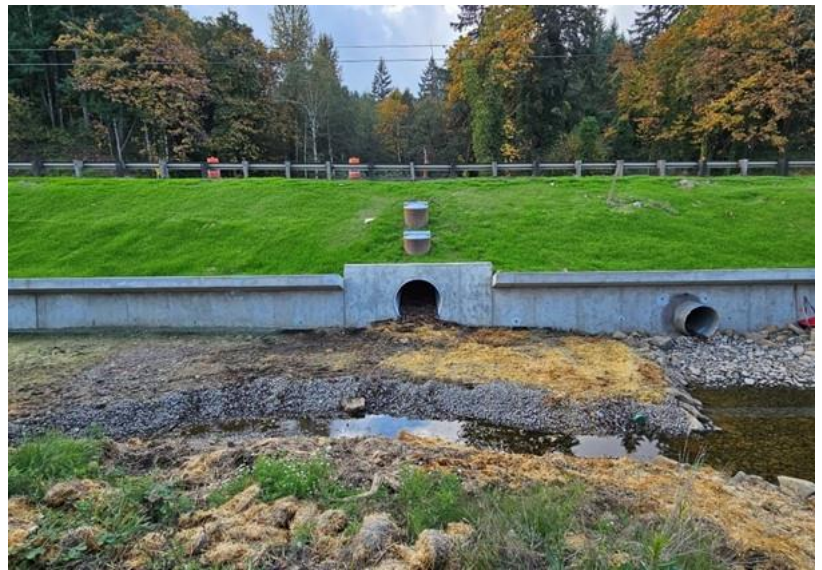
The channelizing wall between the highway and Palensky Wildlife Area was designed to lead Northern red-legged frogs from their wetland breeding areas to the underpass and their upland habitat. Site hydrology was modified to direct all flow towards the culvert (on the right) to prevent water from flowing through the underpass.
