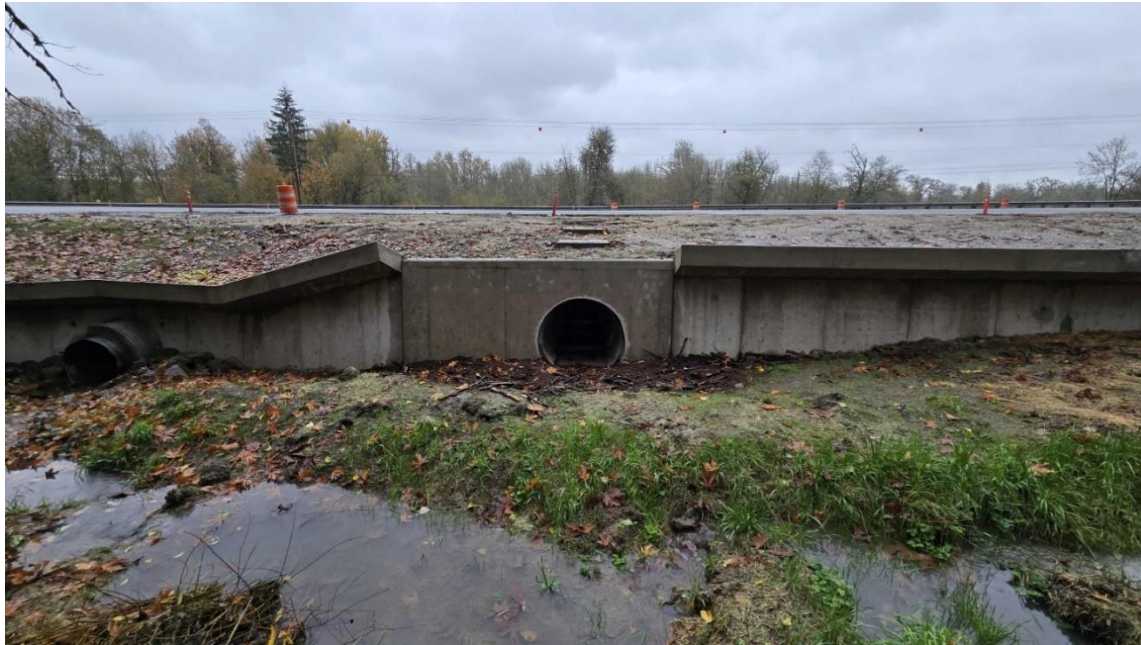
The flare at the top of the channelizing wall was designed to prevent Northern red-legged frogs from climbing over the wall onto the highway, but also prevents frogs from becoming trapped on the highway or road shoulder.
